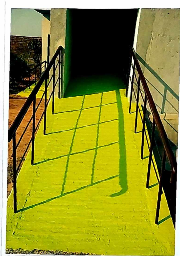
FIRST FLOOR RAMP
